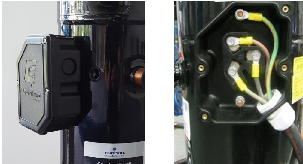
Figure 17: IP54 T-Box and correct electrical installation with cable gland
