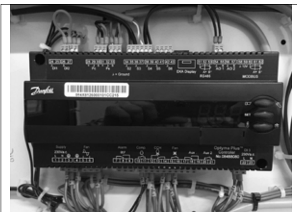
Picture 4 : Normal wiring
